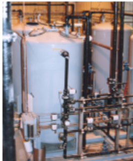
Ion Exchange system for a Superfund site.
